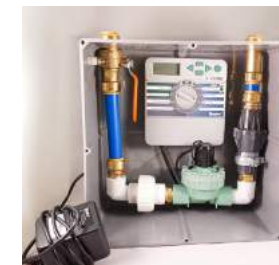
Irrigation Control Unit w/ fertilizer injector system
